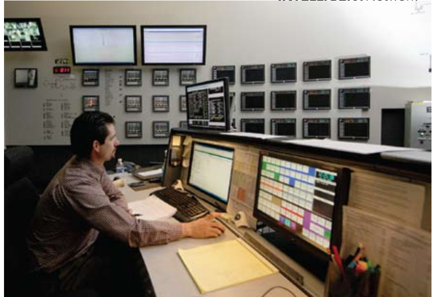
Phasor applications are visually displayed on a large wall monitor at Southern California Edison's Grid Control Center with operator Mario Kiresich keeping watch at the desk.
